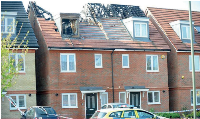
Image 1: inadequate firestop allowed fire spread to neighbouring building
