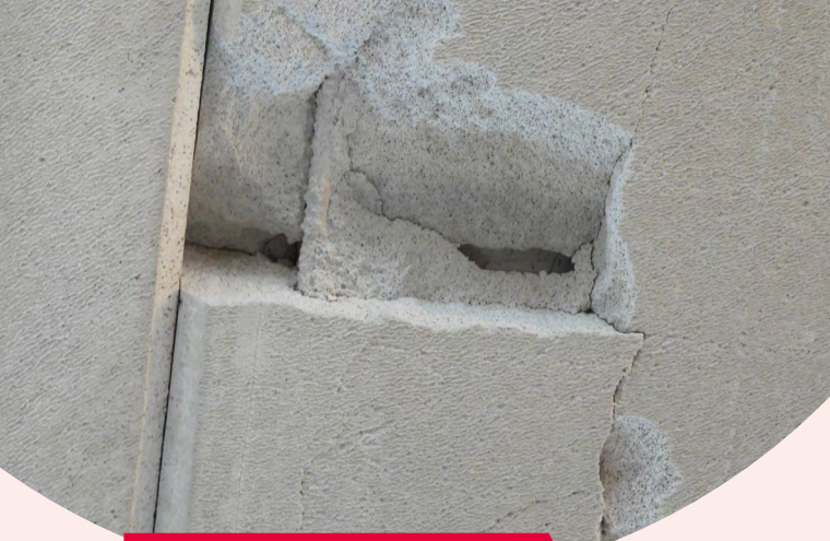
Figure 1: Crumbling RAAC plank
