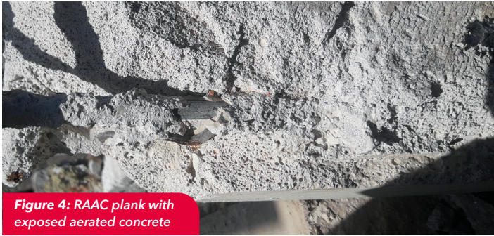
Figure 3: RAAC plank on steelwork who is visible stress fracture
